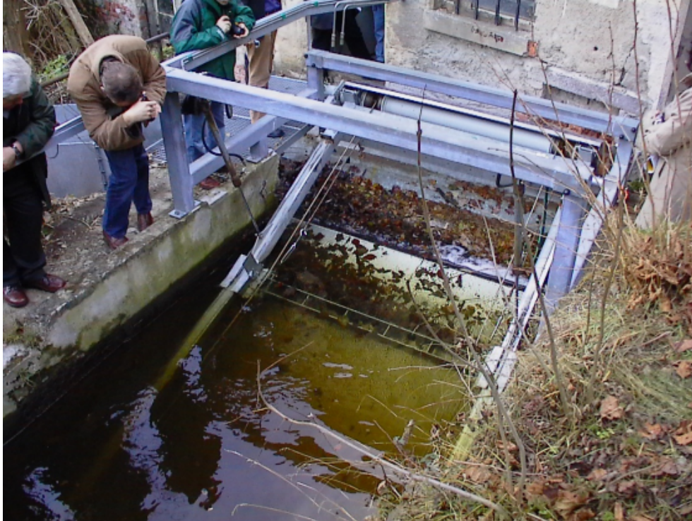
Figure 3.14: Retrofitted inclined wedge wire screen pilot facility (5 mm spacing) with surface bypass and cleaner in an intake channel of a German mini-hydropower plant (design flow: 1.7 m 3 /s) (Photo: Marq Redeker)
