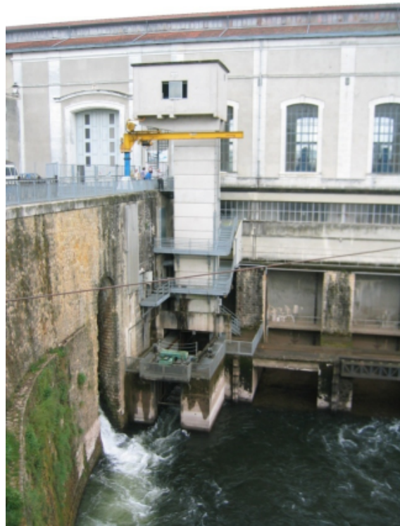
Figure 3.13: Fish lift at Tuilières hydropower station, Dordogne River, France (Photo: Marq Redeker)
