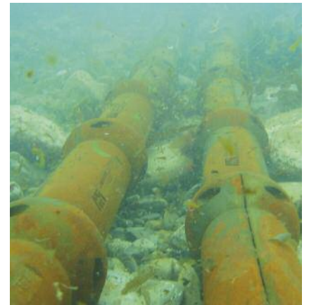
Armoured sub sea cables.
