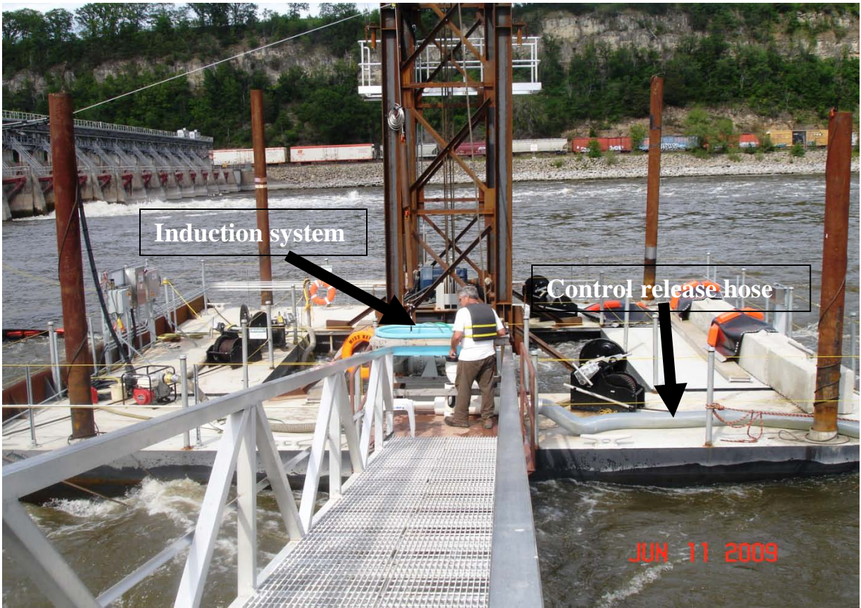
Figure 3-9. Large fish induction system, configured for control releases, located on the HGE hydrokinetic barge.
