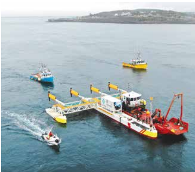
SMEC Plat-I Installation, Grand Passage, NS, photo credit: SMEC
