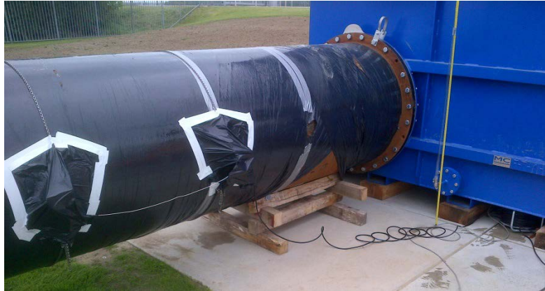
Figure 3: Measurement location transit time flowmeter, located on inlet pipeline.
