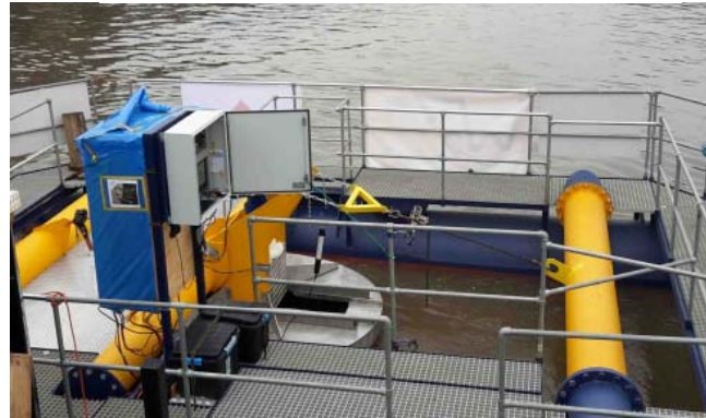
Power recording unit
