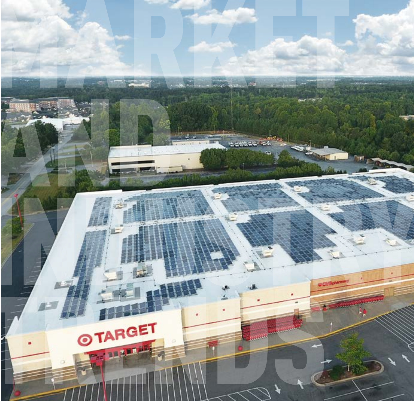
Solar panels on Target store Greenville, South Carolina, United States
