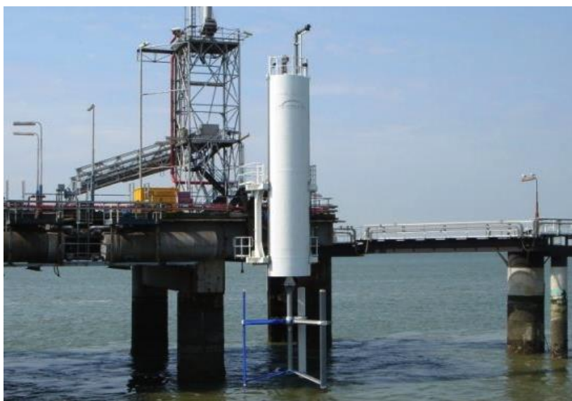
Figure 8 C-Energy project in the Westerschelde (2009), a 30kWp grid-connected vertical axis tidal turbine at a jetty of Zeeland Refineries near Borselle.
